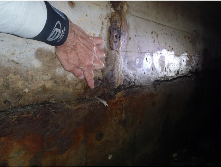
13) Sta 145 Cold Joint with Outside Material Entering
