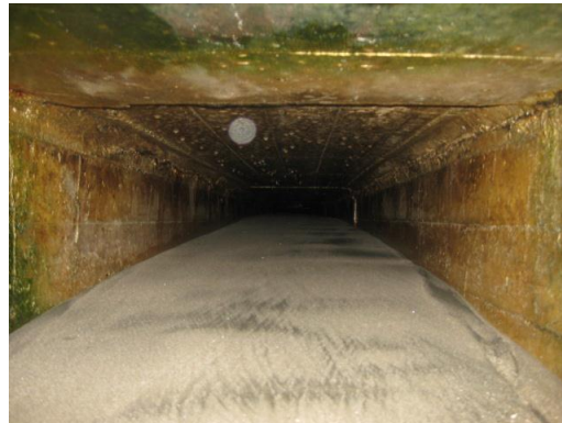
8-Inside Flume Filled with Sand Near Outlet 5pm
