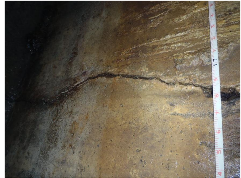
6) Sta 16 Left Side Horizontal Crack
