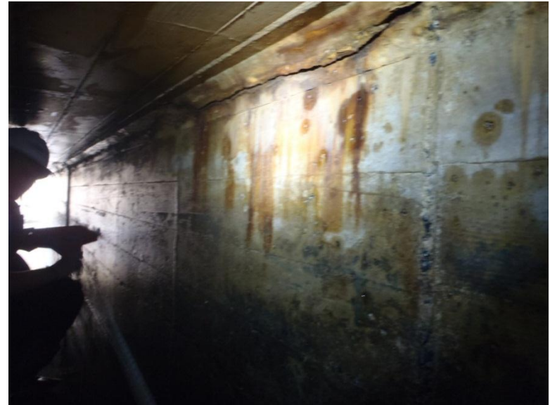
16) Right Side Crack at Top
