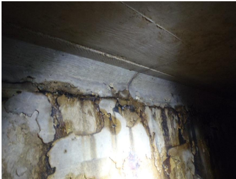
7) Sta 30 Left Side Longitudinal Cold Joint/Crack
