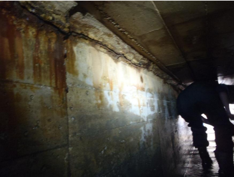
15) Sta 199 Left Side Crack at Top
