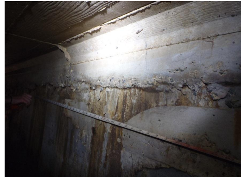
8) Sta 51 Right Side Cold Joint/Crack
