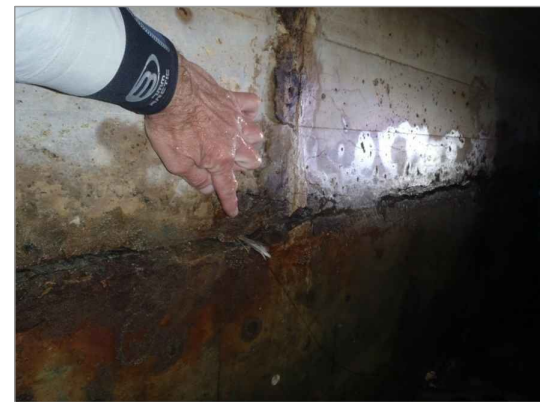
STA 1+45 COLD JOINT WITH OUTSIDE MATERIAL ENTERING
