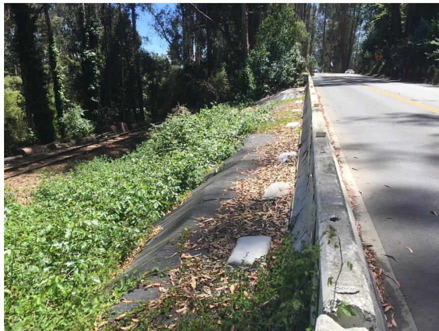
Photo 1. Slope Damage Along Park Avenue, taken July 7, 2018
