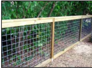
NEW DOG RUN FENCE: 4' TALL WELDED WIRE MESH PANEL WOOD MEMBERS: STAIN PLATINUM GRAY
