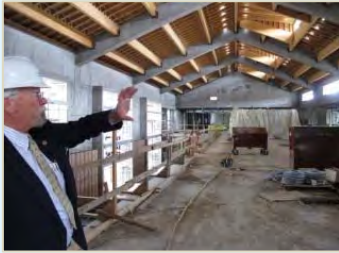
In this photo, Dan is leading the City Council on a tour of the partially completed new facility.
