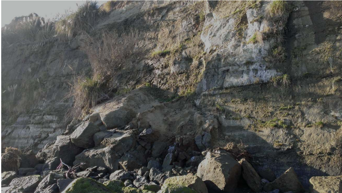
Coastal Bluff Erosion Debris on Beach as it Existed on November 7, 2014 at the Property
